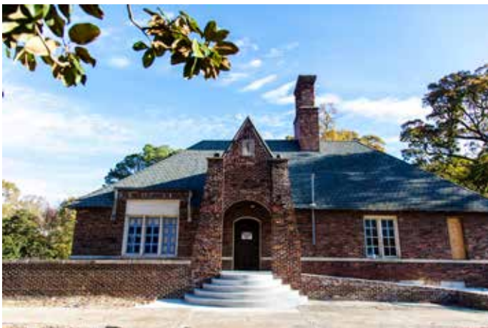
The golf clubhouse renovation includes an overhaul of the entrances, steps, and back terrace.
